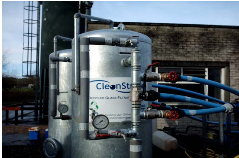
Figure 3.. The full-scale filters as installed at Malton
