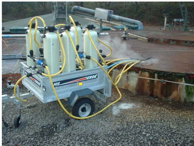
Figure 2. The five trailer-mounted filter units in the pilot trials
