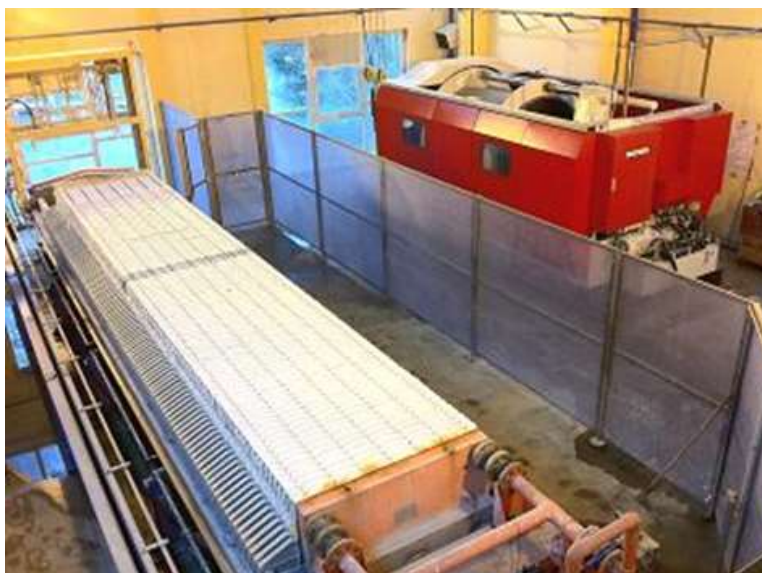
Figure 7: Dewatering workshop with the filter press and the Bucher press
